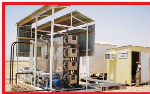
Heating skid and control cabinets
